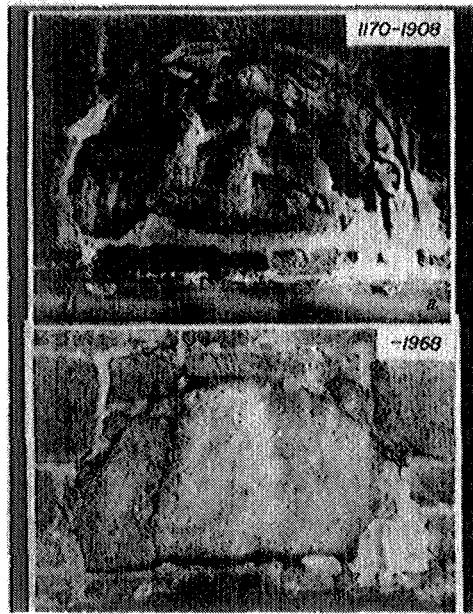
Figure 3. Rapid decay towards total destruction of relief on tympanon of parish church in Opherdicke, near Unna, Westfalia. Destruction was severe in 1893, after 600 years of exposure, but catastrophic within the last 80 years. The rate of weathering of Figure 2. appears to apply here too. Stone is Soest Greensandstone with 65% calcite. Photos and information were supplied by Mr. Schmidt-Thomsen, Landesdenkmalamt Westfalia-Lippe, Germany.
